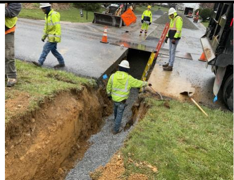
Force Main at Monticello Drive and Lincoln Ave Intersection
