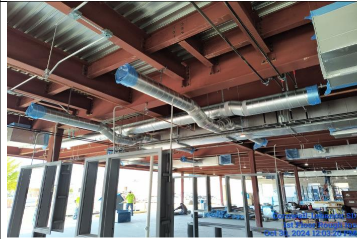
1st Floor HVAC
