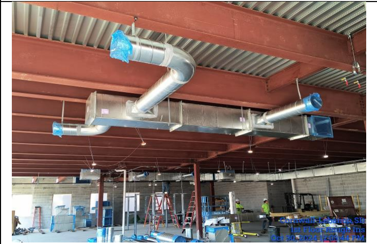
1st Floor HVAC
